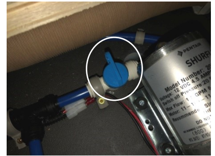
Fresh water drain valve
