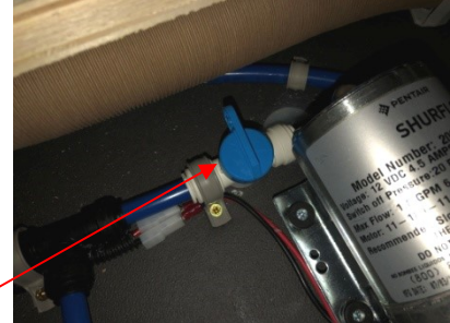
Fresh water drain valve
