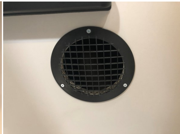
Cold air intake grill
