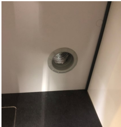
Air vent for the warm air
