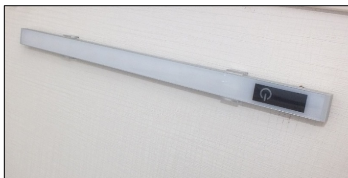
Lighting strip on the bathroom/toilet ceiling with sensor button
