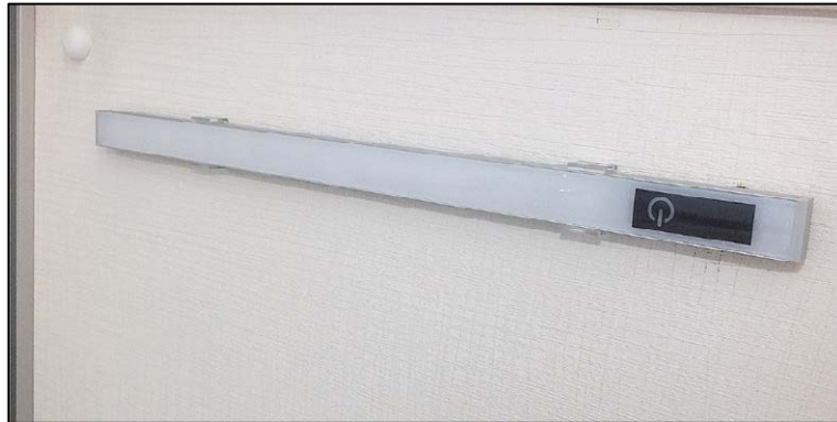
Lighting strip on the bathroom/toilet ceiling with sensor button
