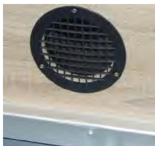
Cold air intake grille
