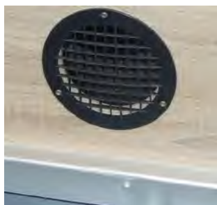
Cold air intake grille
