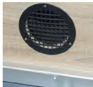
Cold air intake grille
