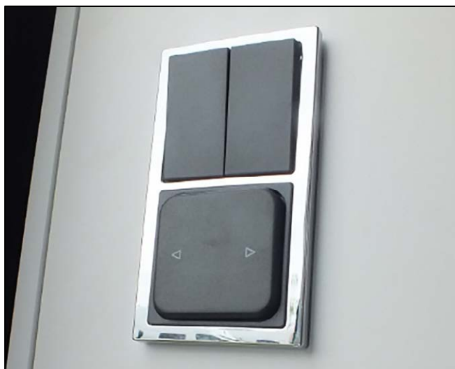
Switch on the kitchen cabinet in the entryway
