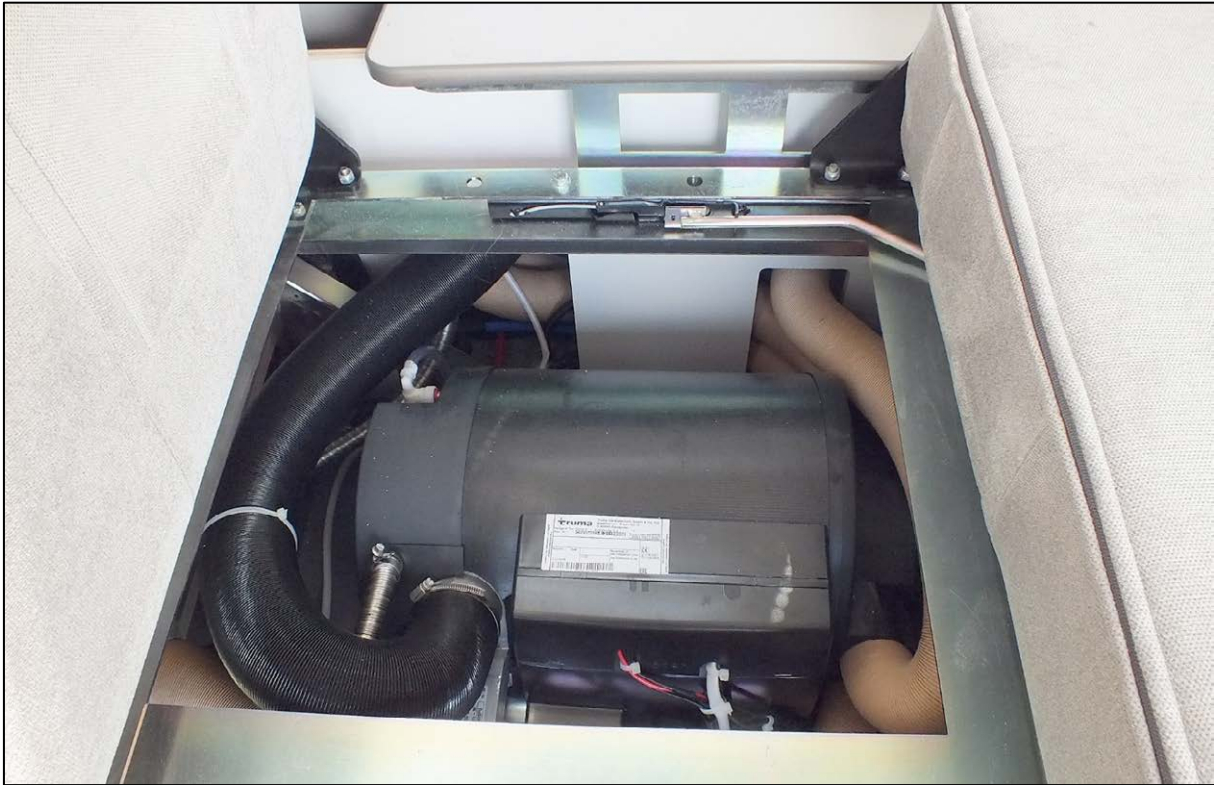
Heating system under the bench seat
